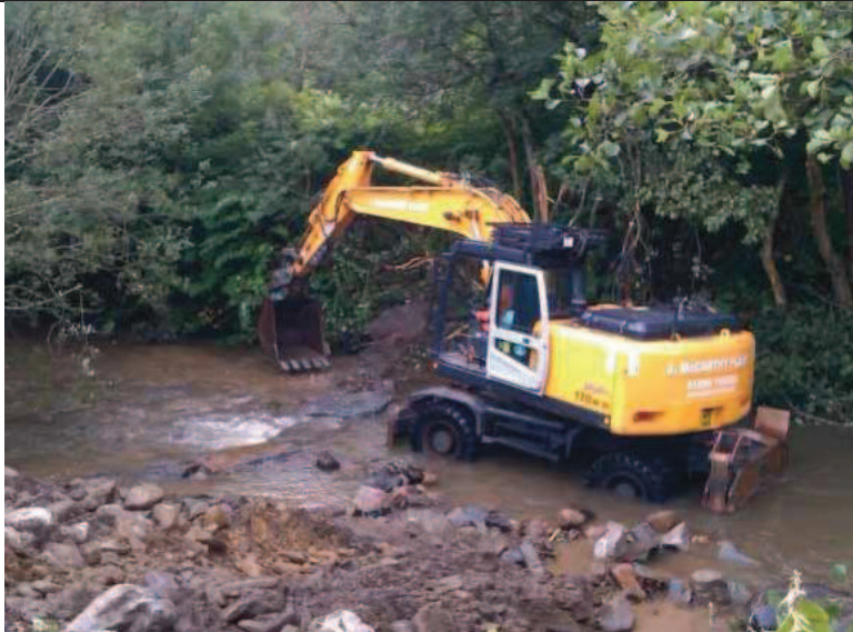
Installation of a pre barrage at Penmaen weir to enable salmon to pass upstream
